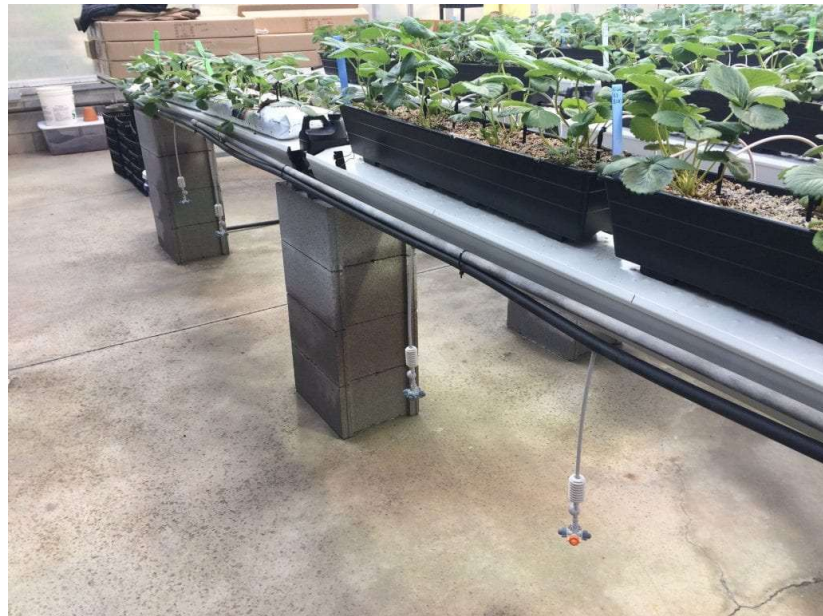
Figure 5. An under-bench mist system to increase nighttime humidity. Image: Chieri Kubota, Ohio State University, https://u.osu.edu/indoorberry/tip-burn/
