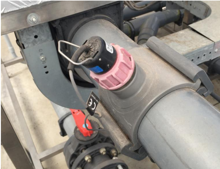
Figure 4. In-line pH probe plumbed into the irrigation line, measuring the pH of the irrigation water and fertilizer solution going to the crops.
