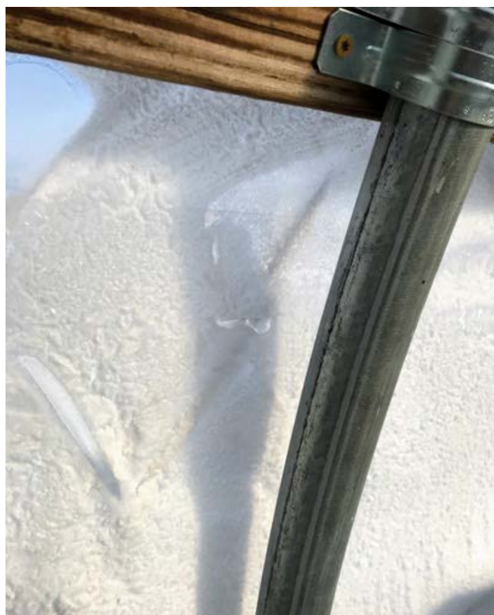
Figure 10. An inflation fan installed incorrectly, pulling air from inside the greenhouse causing condensation to occur in between the layers and freezing. Photo credit: W. Garrett Owen
