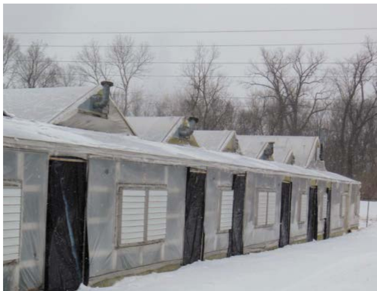
Figure 5. Greenhouse exit doors covered and sealed to prevent heat loss and cold air from leaking into the greenhouse. Photo credit: W. Garrett Owen
